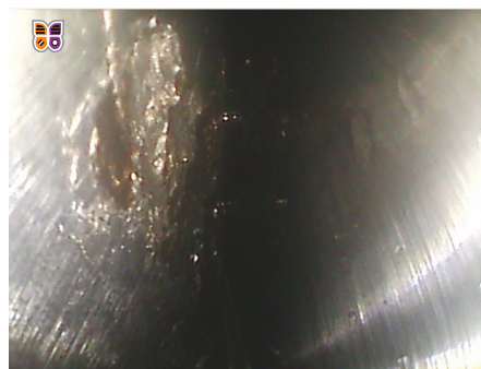
Inspection found pitting on generator side IMS bearing
